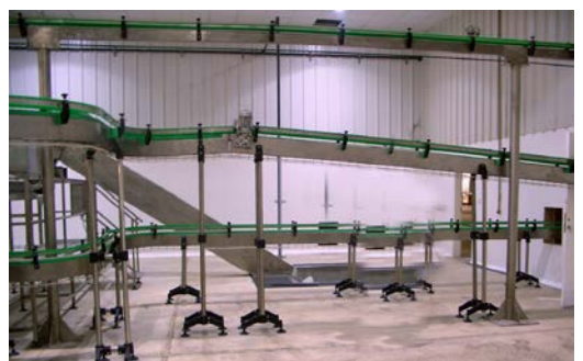
OVER HEAD CAN CONVEYOR
