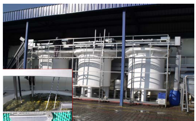
FULL AUTOMATED PICKLES DESALINATION SYSTEM
