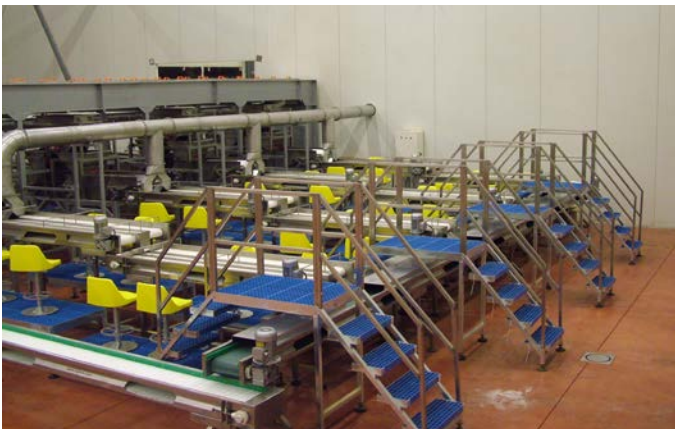
PLC CONTROLLED DISTRIBUTION W-BUCKET ELEVATOR
